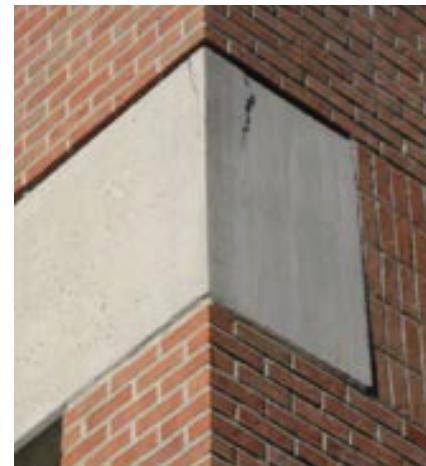
Typical corner settlement and cracking
