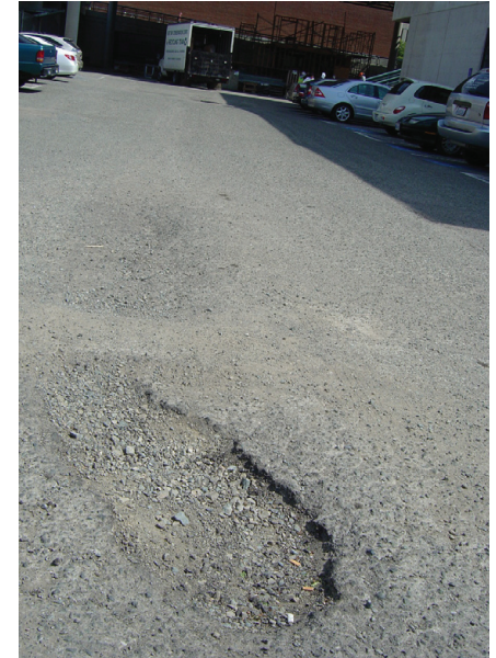
Lower level asphalt paving with tripping hazards
