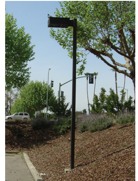
Perimeter light fixture
