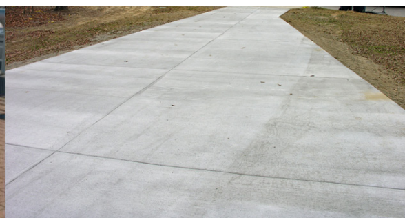
General campus paving Standard gray concrete, light broom finish Concrete to contain minimum 15% slag, 15% fly ash to meet LEED standards.
